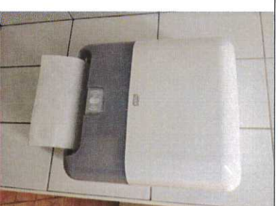
'Touchless' hygiene equipment in place
