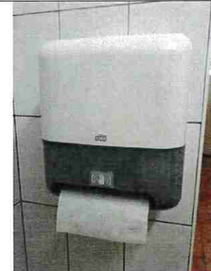
'Touchless' hygiene equipment in place
